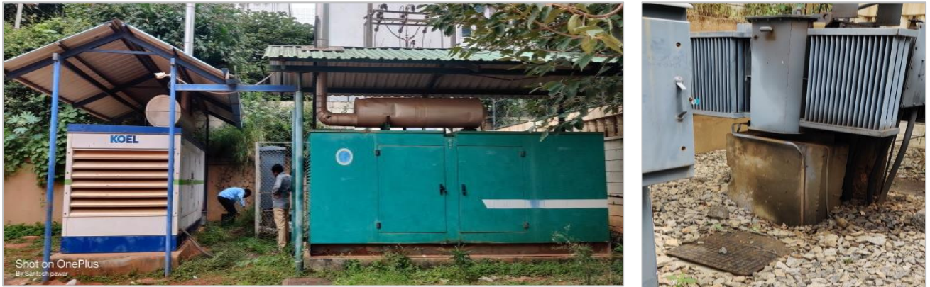
Investigative parameters – Ecological Management – Diesel Generator, earth pit areas for backup measures
